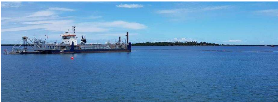
Figure 11: Example of suction dredge with dredge pipe off stern. Source: Fogafale Lagoon Shore Reclamation Preliminary Environmental Assessment
