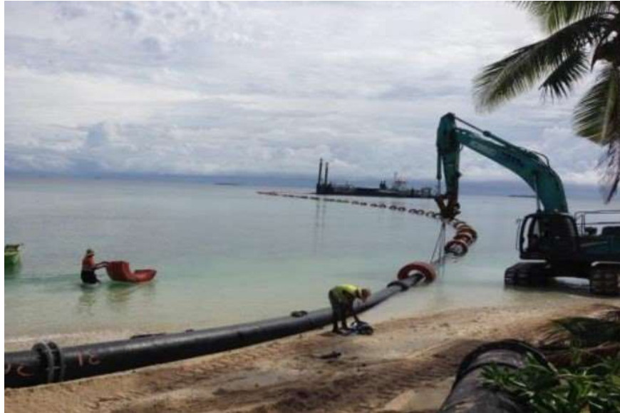
Figure 12: Dredge pipeline on shore for the Tuvalu Borrow Pit Reclamation Project. Source: Hall Contracting
